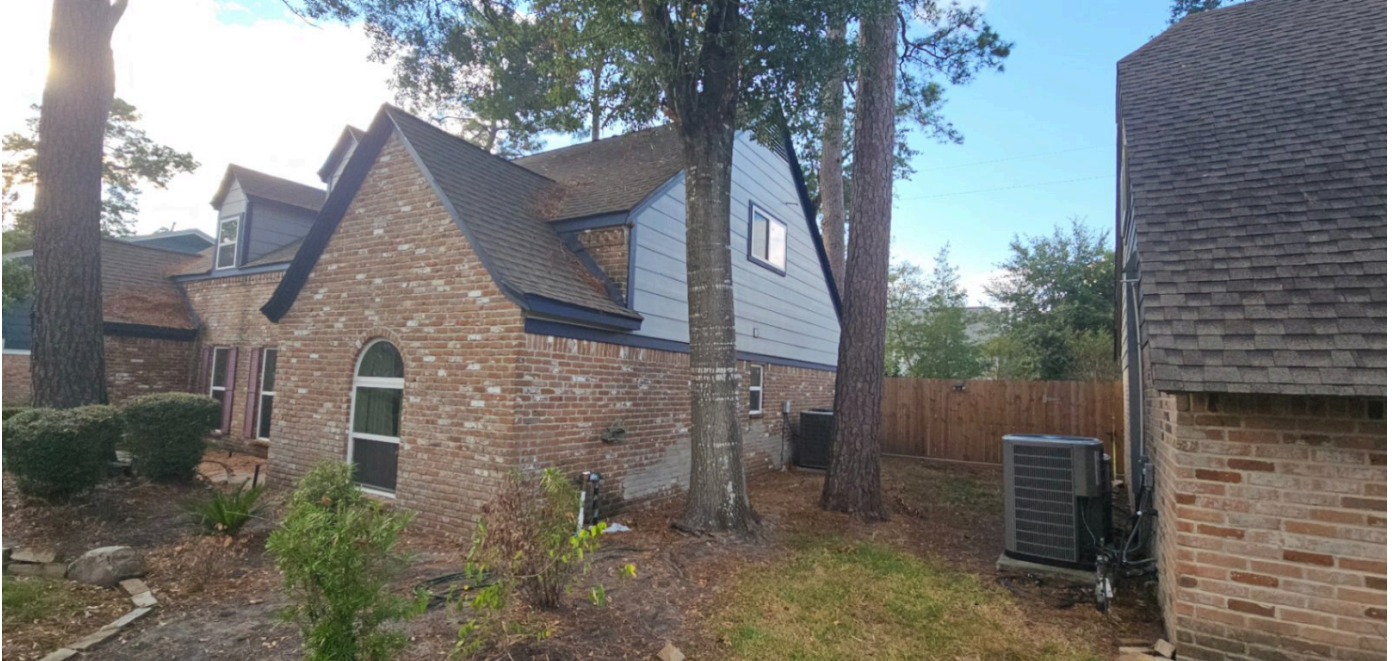
Exterior Wall Hazard - Other
