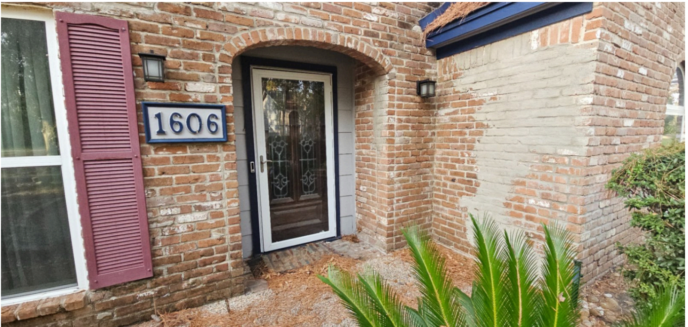
Exterior Wall Hazard - Other
