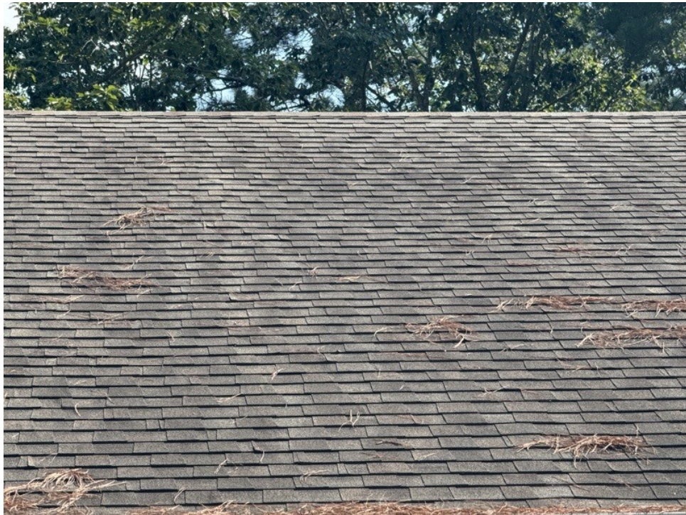
Roof verification, Left, Dwelling, Roof, Front, Sagging/Bowed
