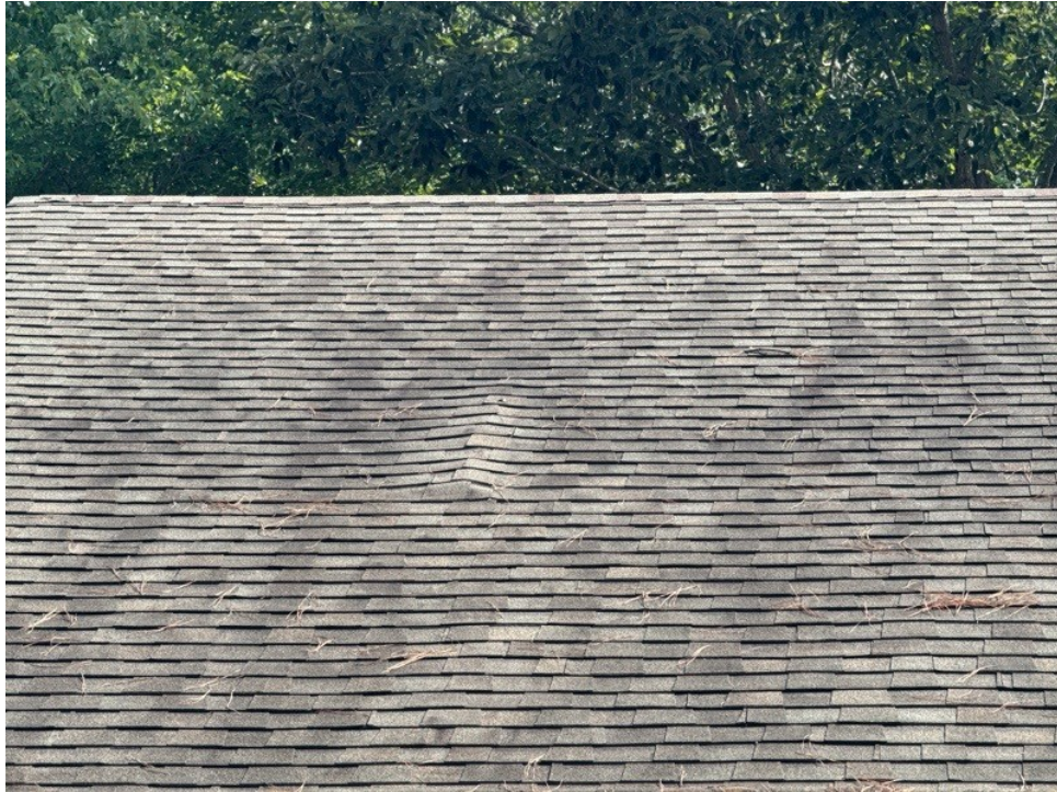
Roof verification, Left, Right, Dwelling, Roof, Front, Sagging/Bowed
