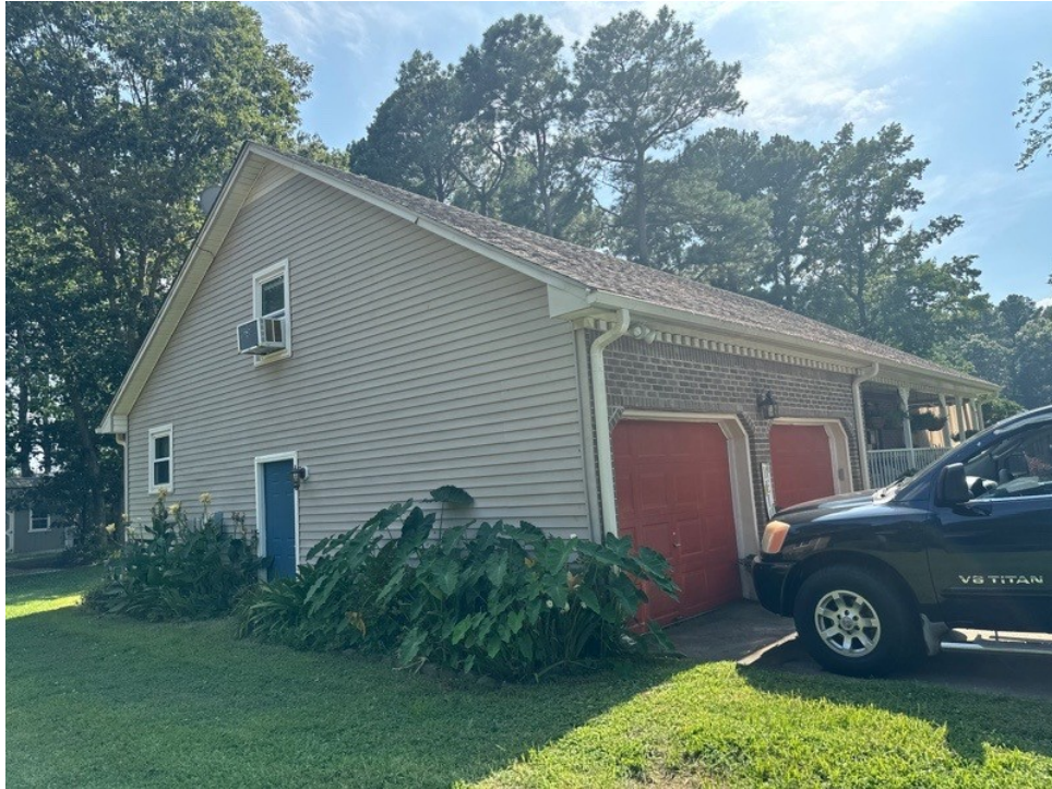
Left view, Dwelling, Gutters, Front, Downspout discharges onto walkway/driveway
