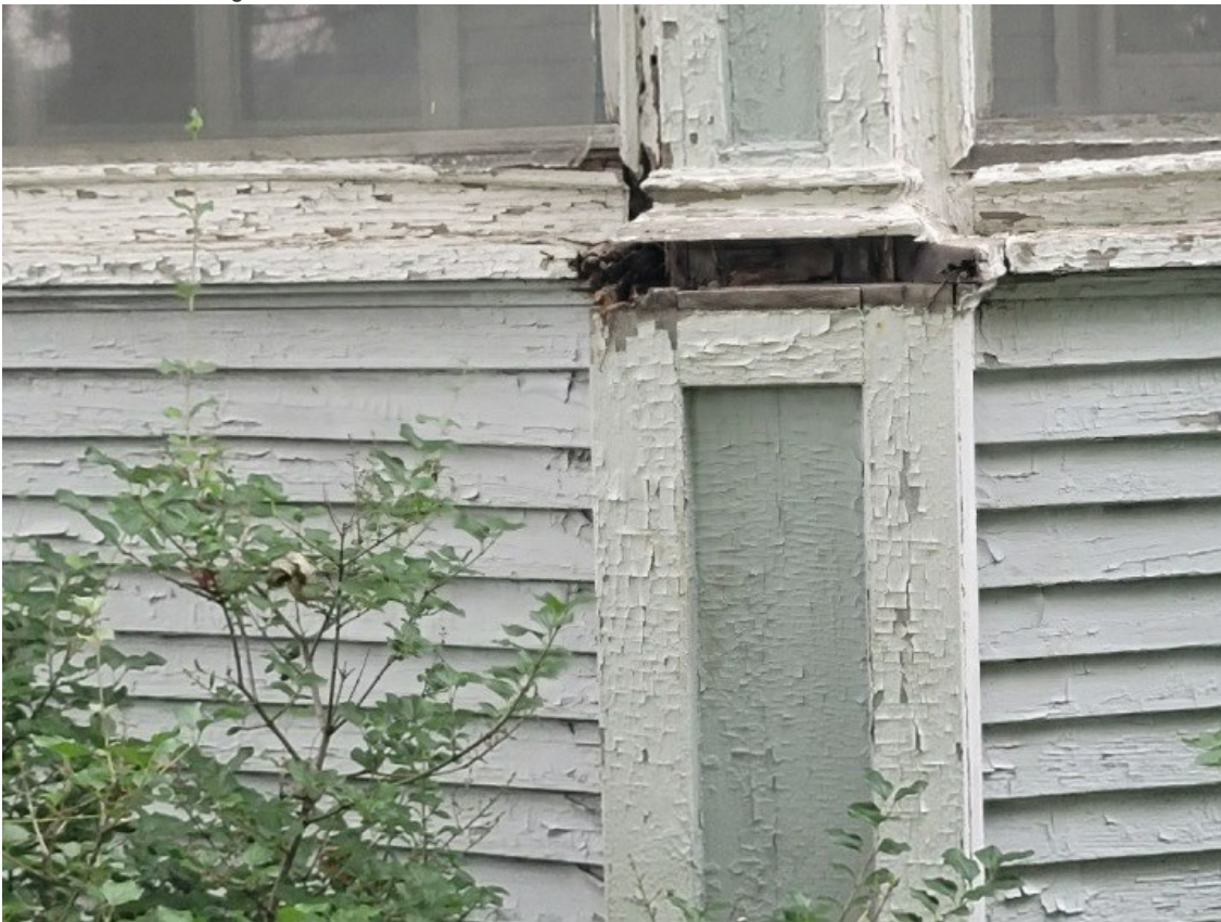
8Exterior Wall Hazard
