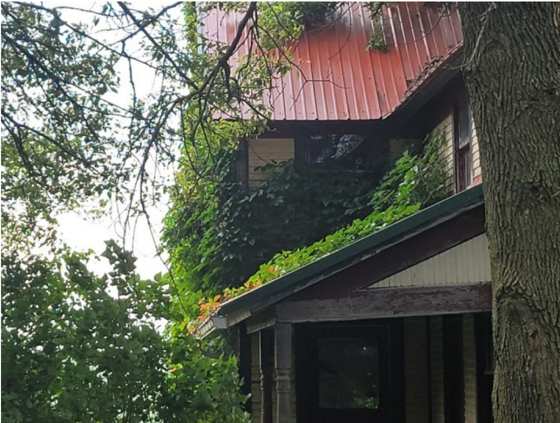
33 Detached Structure Hazard
