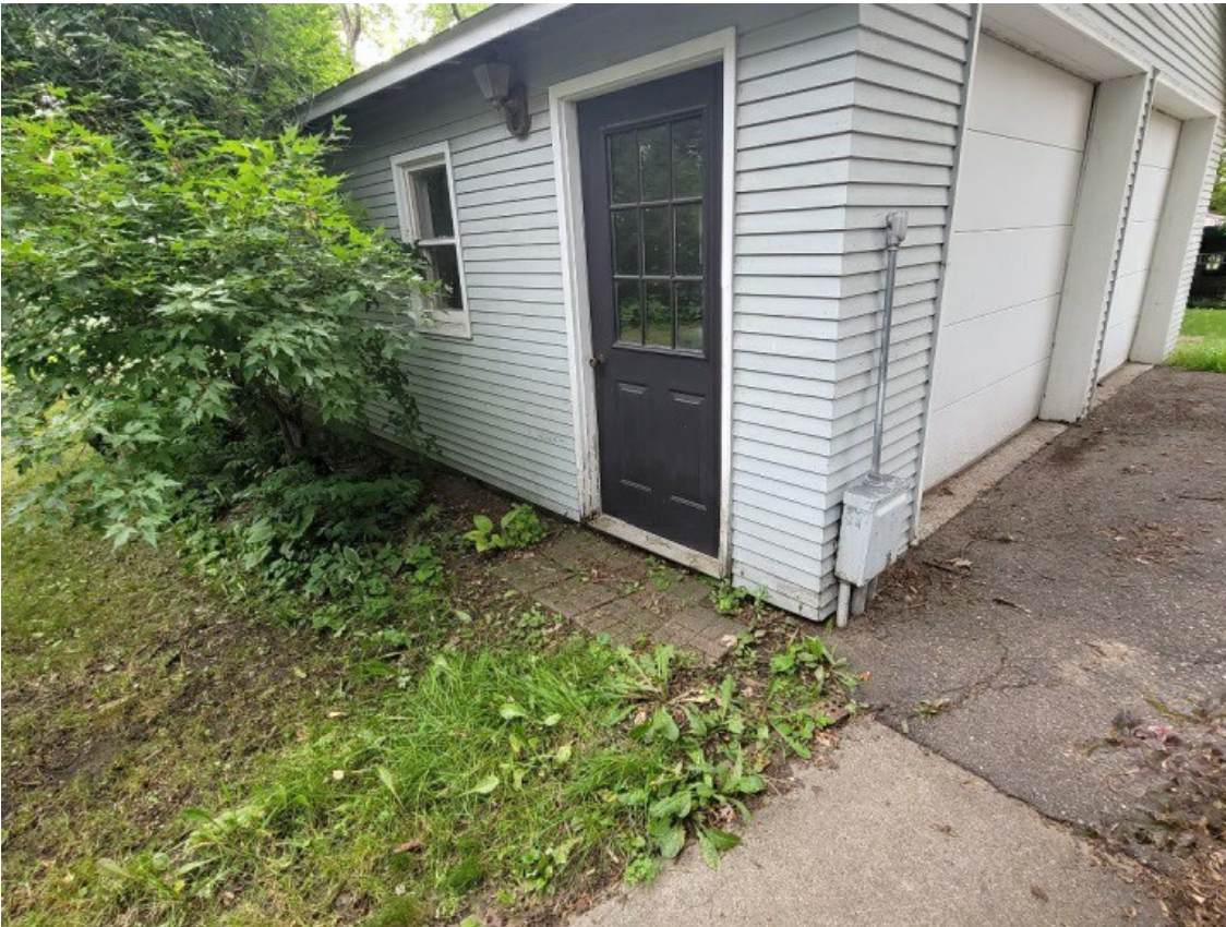
15 Detached Structure Hazard
