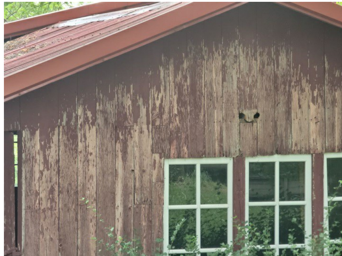
26 Detached Structure Hazard
