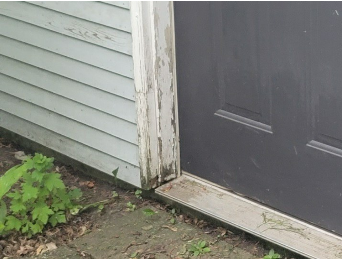
14 Detached Structure Hazard
