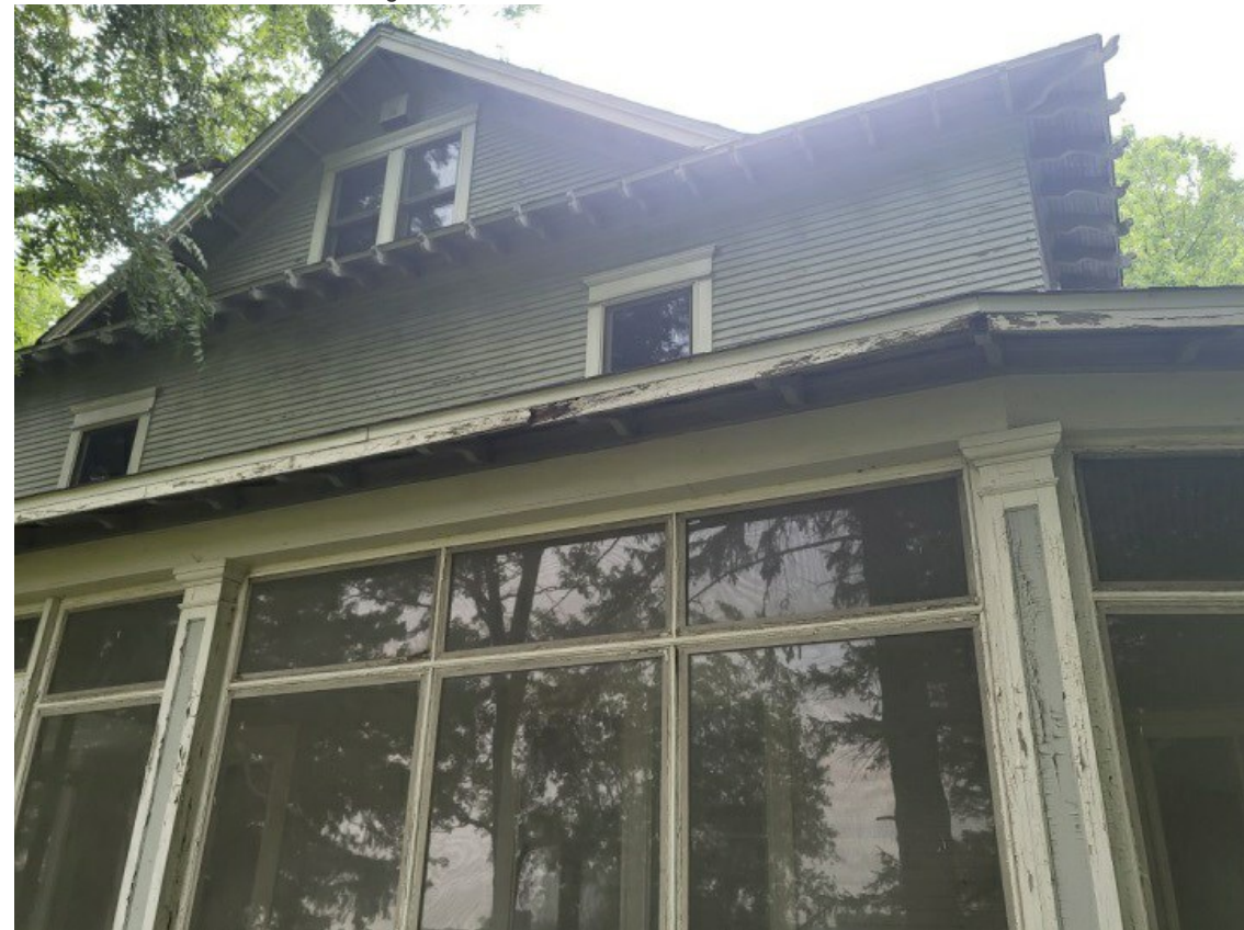
24Soffit, Fascia, Eaves & Overhangs Hazard
