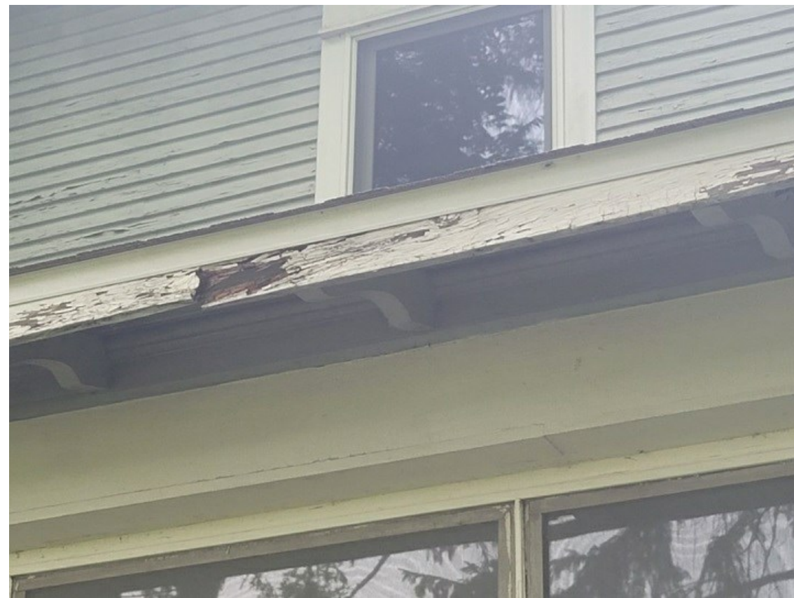
23Soffit, Fascia, Eaves & Overhangs Hazard
